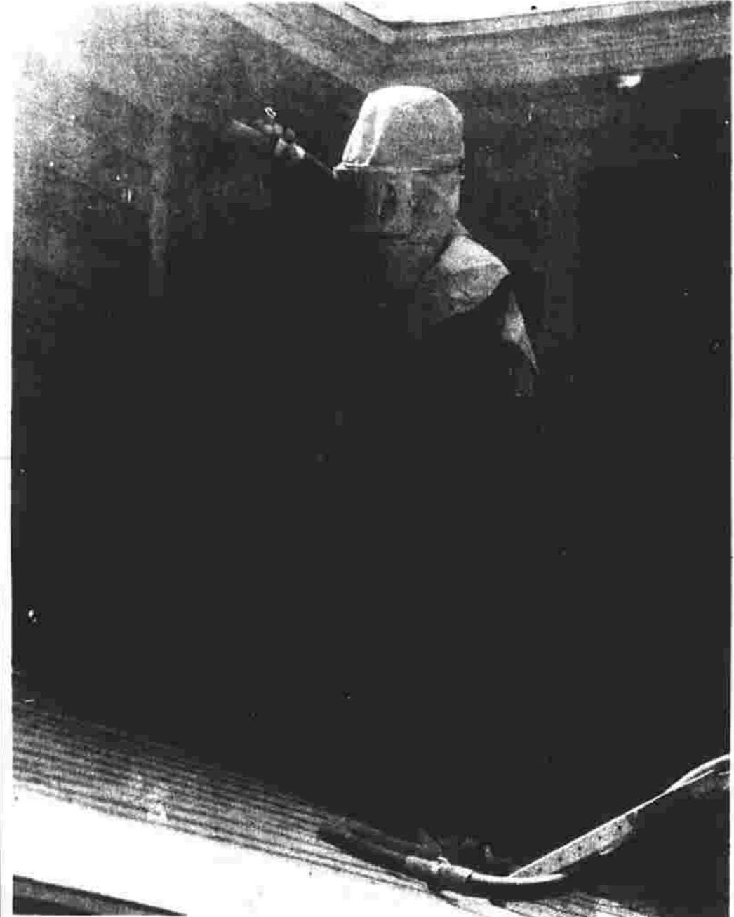
Evan Nay, working for Simsbury Sand Blasting, is surrounded by airborne particles as he sandblasts the exterior of a house at 182 Vernon St. The one-day job was done last week.
